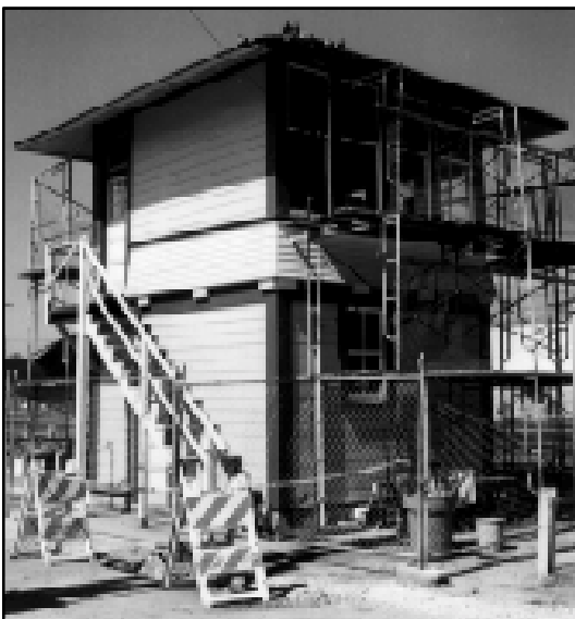
RESTORATION WORK CONTINUES — Work on the Santa Clara Interlocking Control Tower, located at the north end of the Caltrain parking lot of the Santa Clara Depot, has continued during the summer months. Work parties used one full weekend each month to make the progress that will soon result in the removal of the scaffolding from around the historic structure.
